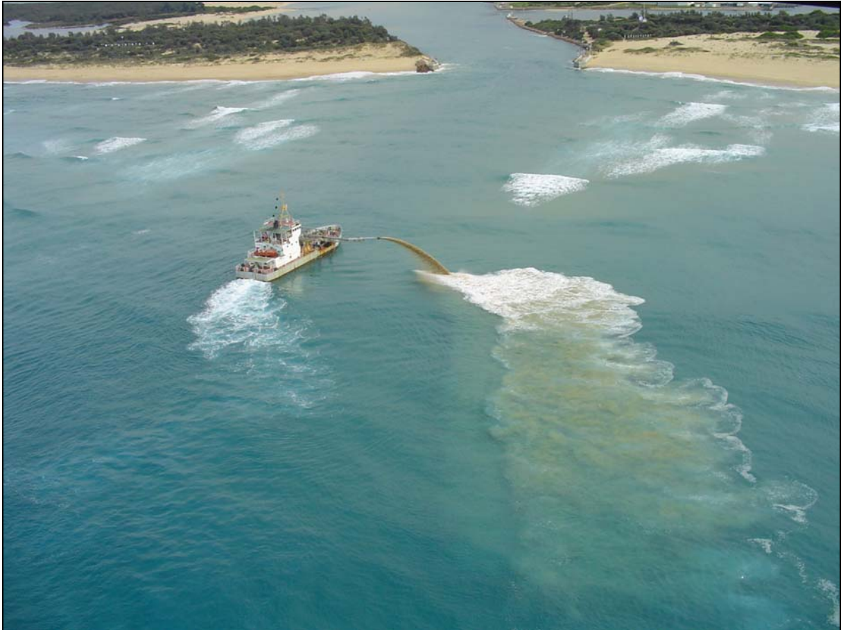
Fig. 6 The Gippsland Ports side-cast dredger April Hamer during dredging operations at the ebb-tide delta in Bass Strait on an ebb-tide. Source: Wheeler (2005)
